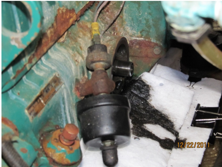
Figure : Approximately ¼ cup of oil escapes upon oil filter removal. Oil absorbent pads caught most of the escaped oil. Photo shows how a larger binder clip is used to secure pad and cardboard platform to engine bed.
