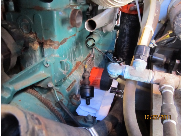
Figure : Oil absorbent pads mounted on cardboard platform shown under filter prior to removal. Extra pads have been folded and placed beneath filter. This photo shows how access was improved by following steps A thru E.
